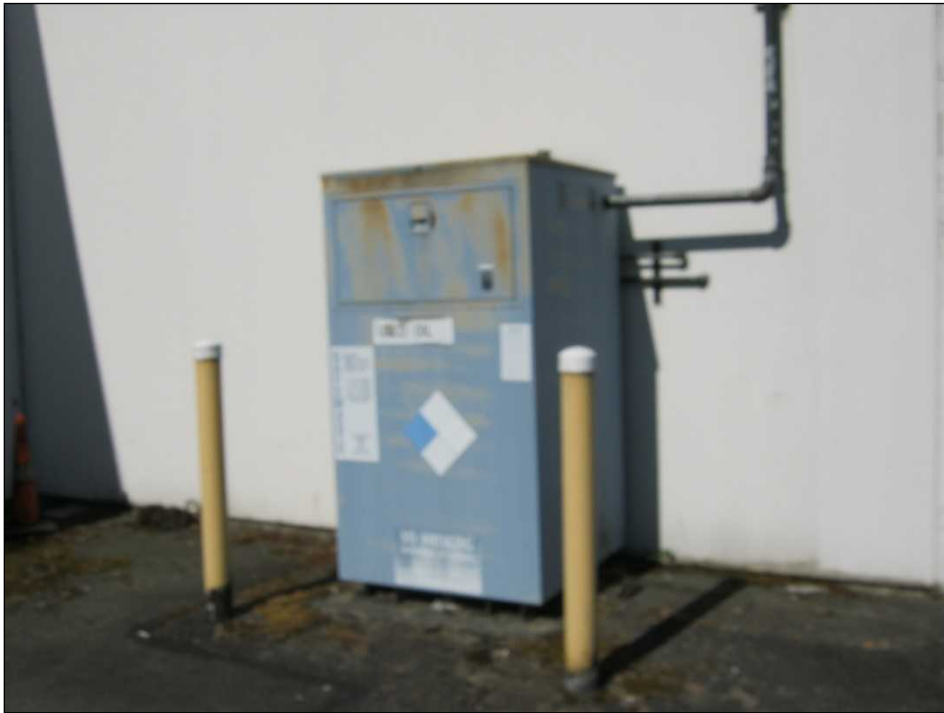
15. Waste oil AST (reportedly out of service)
