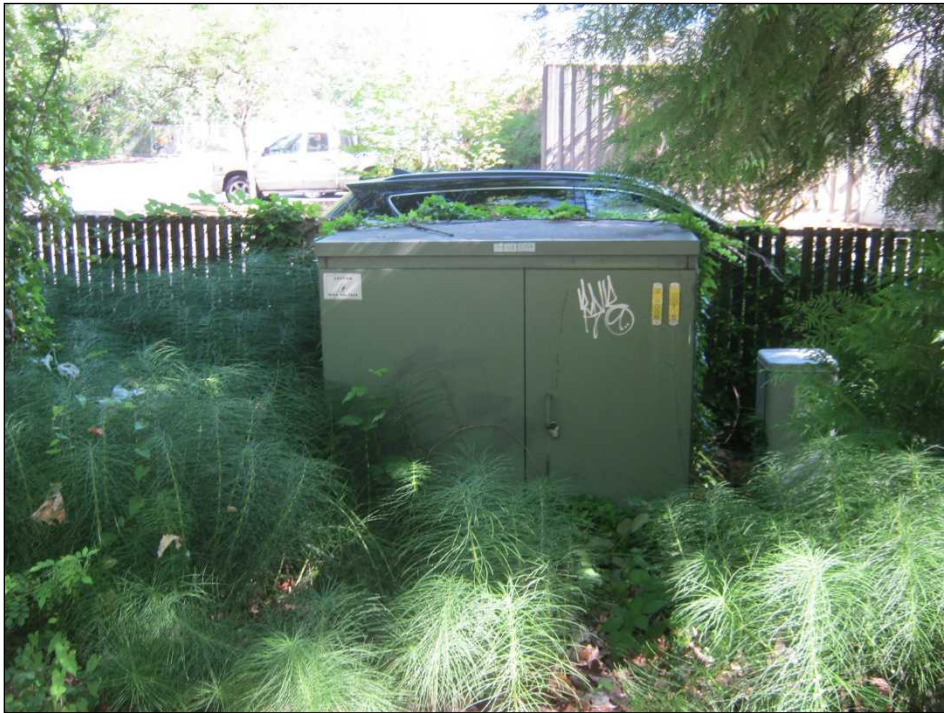
21. On-site electrical transformer
