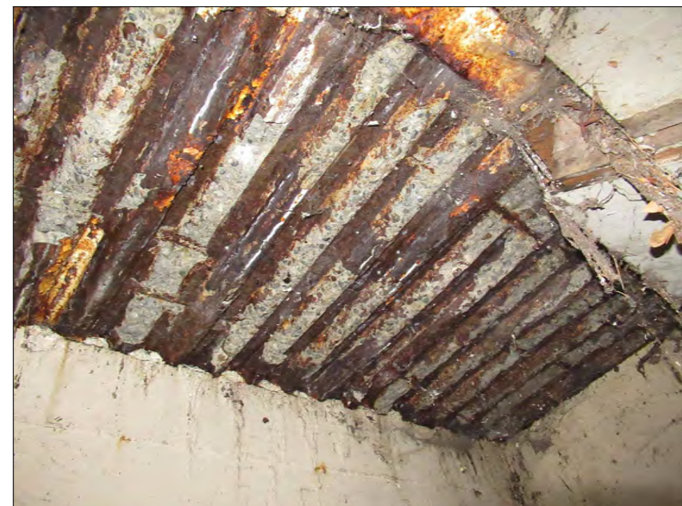
CORRODED STEEL FAN DECK BELOW LANDING
